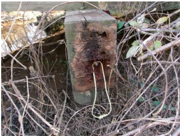
Rot in end of Bent 2 left cap
