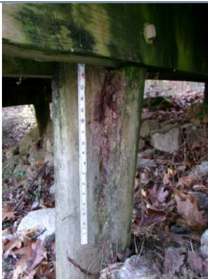
Split in Pile 1 at Bent 2
