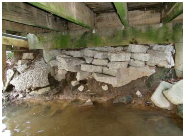
Rip rap/stacked concrete at Bent 4
