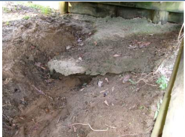
Erosion channel extending out from under concrete overpour at Bent 1 endroll
