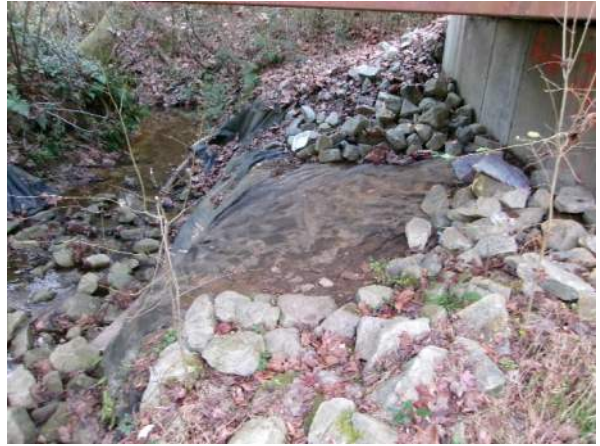
Displacement of rip rap at both abutment endrolls
