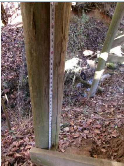
Split in Pile 2 at Bent 6
