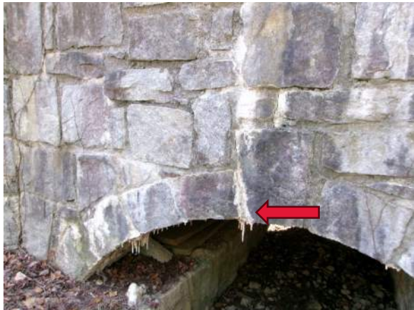
Typical of heavy efflorescence in masonry headwall
