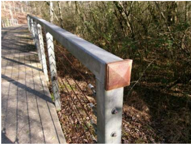
Surface corrosion of handrail end cap
