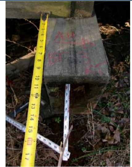
Rot in end of Bent 3 right cap
