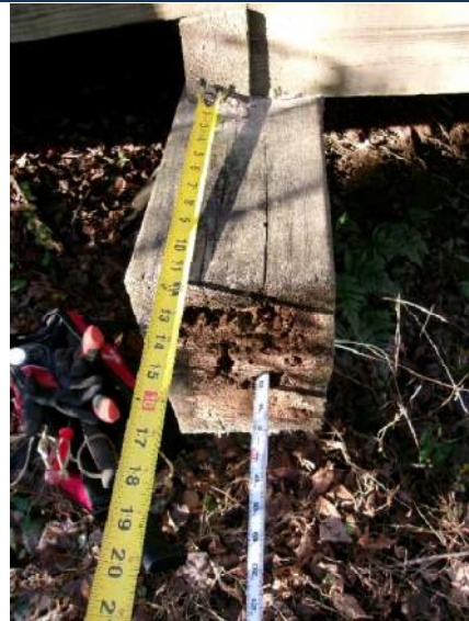
Rot in end of Bent 2 right cap
