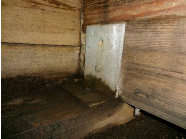
Dirt build up along top of Bent 1 cap that is retaining moisture
