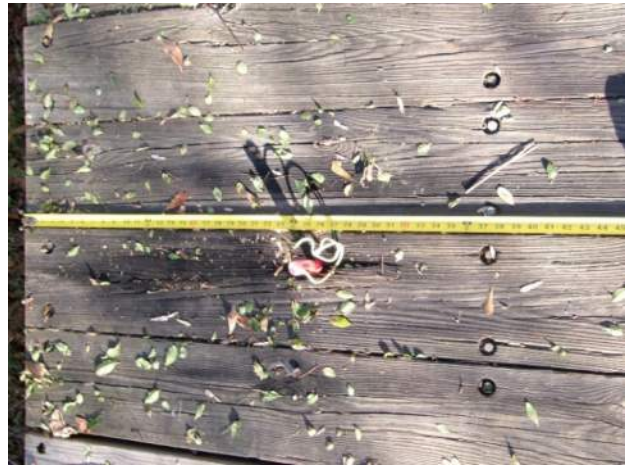
Typical of deck board with splits and rot
