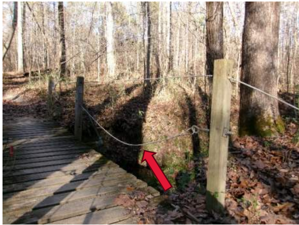
Bottom handrail cable loose
