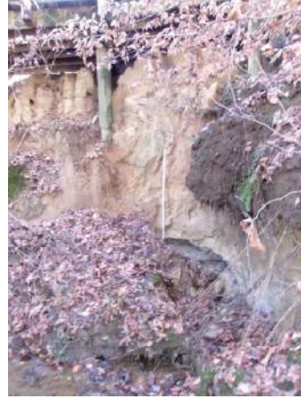
Soil failure at Bent 7 (Pile 2 at Bent 7 shown)
