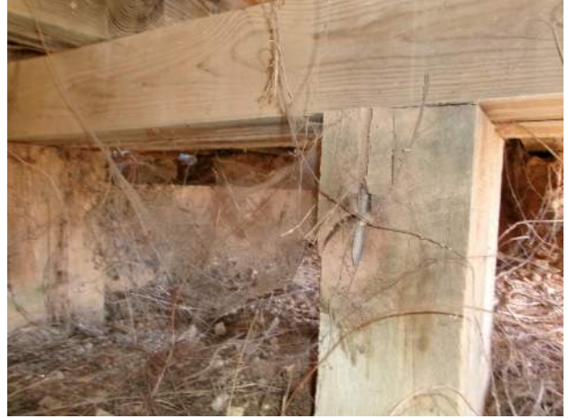
Nail protruding from back face of Column 3 at Bent 5
