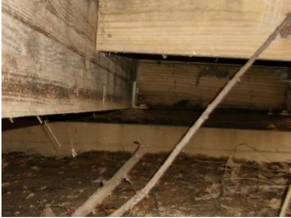
Debris build up along top of Bent 1 cap
