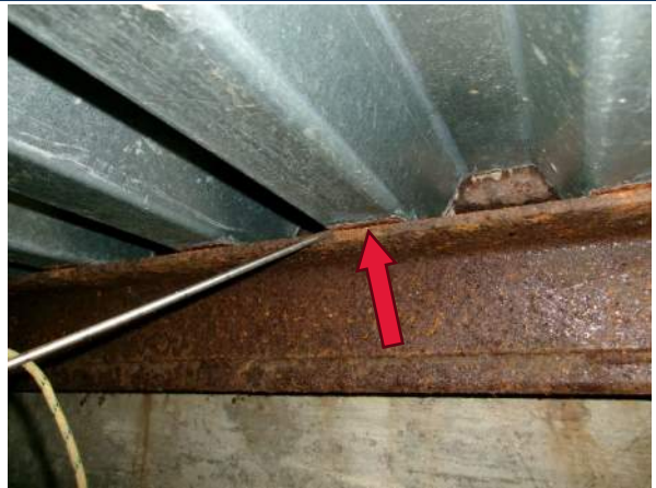
Corrosion forming on bottom of metal deck forms at contact points with weather steel members
