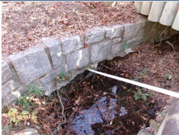
Void and scour hole just down stream from bridge (right masonry wall if looking downstream)
