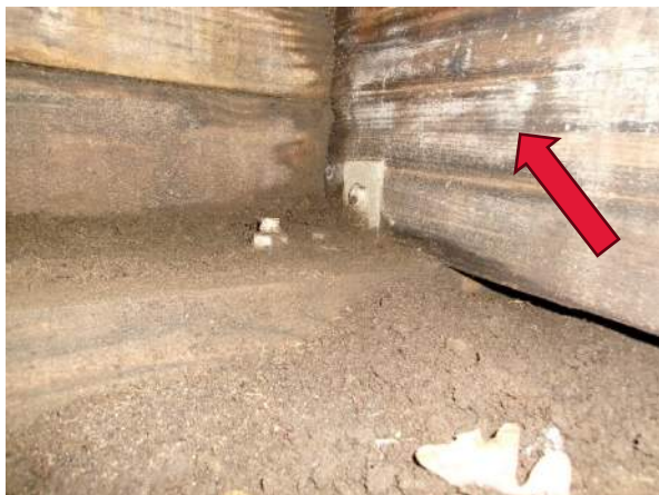
Corrosion forming along edges of steel angle at Bent 5, note the white mold
