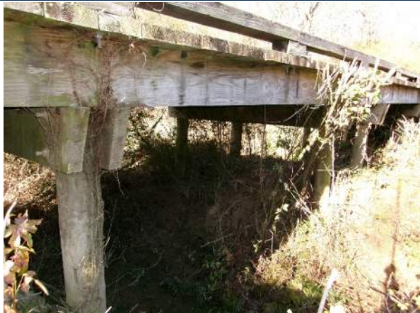
Vegetation growing on and under the bridge in Spans 1-6
