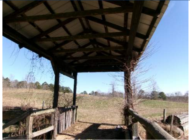
Typical of roof structure and vines growing on bridge elements
