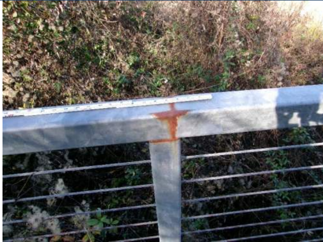
Surface corrosion on top of handrail and around welds
