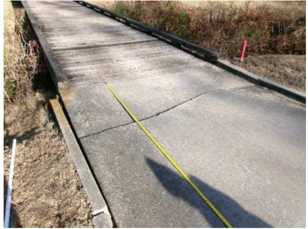
Crack in approach span at Bent 1
