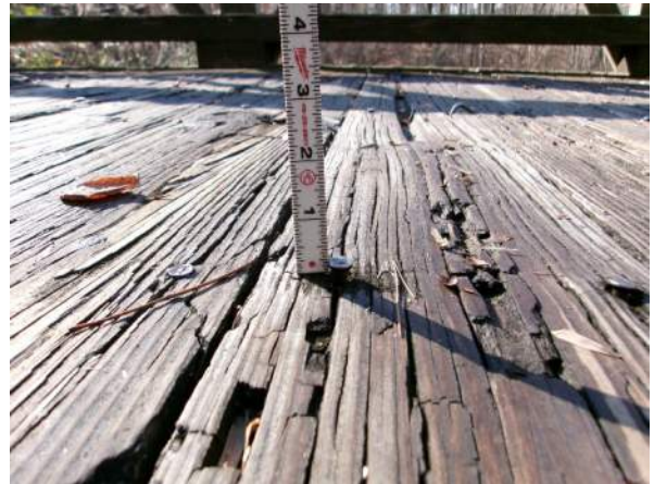
Nail head protruding above deck board, typical
