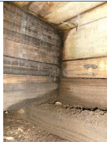
Dirt build up on top of Bent 5 cap
