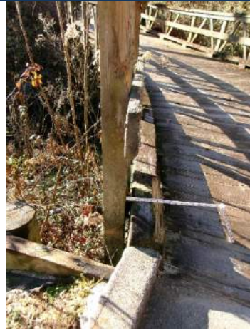
Vertical post of hand rail at Bent 1 pulling away from bridge deck from possible impact
