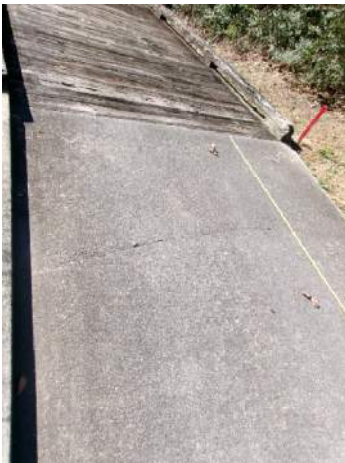
Crack in approach slab at Bent 27
