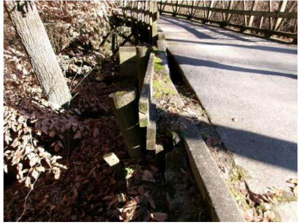
Timber wing wall failing at Bent 8 right (looking back)
