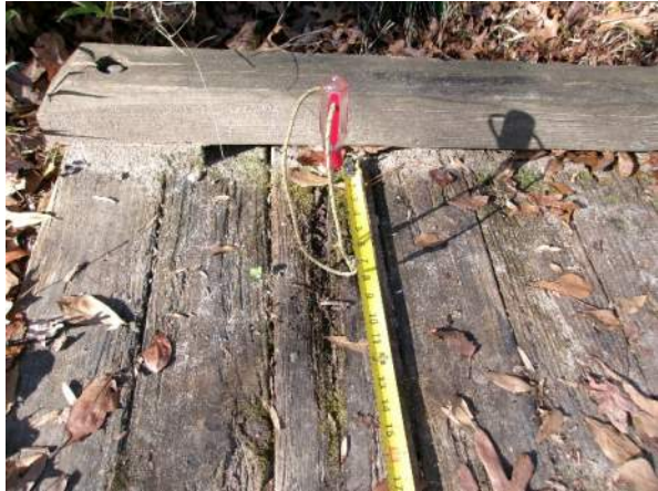
Rot and section loss in deck board along left brush curb at beginning of structure
