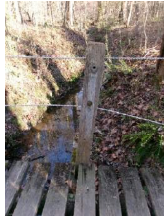
Vertical 4"x6" cable support at midspan, note it is not plumb and can move
