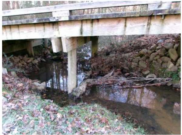
Debris build up on Bent 4
