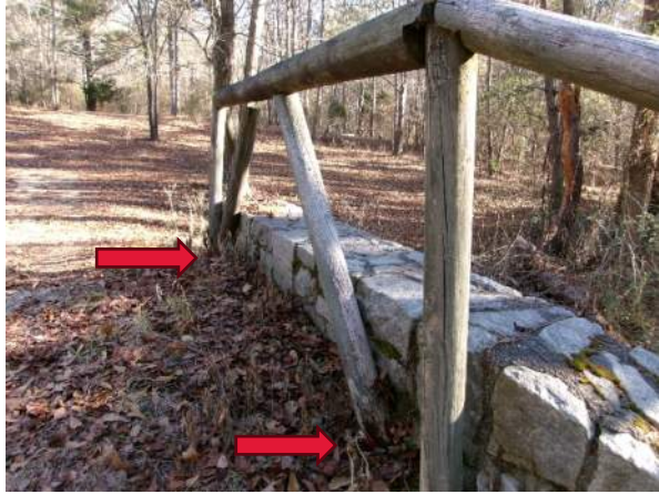
Section loss in handrail members at groundline along right side of culvert
