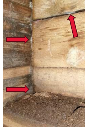
Dirt build up along top of Bent 1 cap, note the white mold growth
