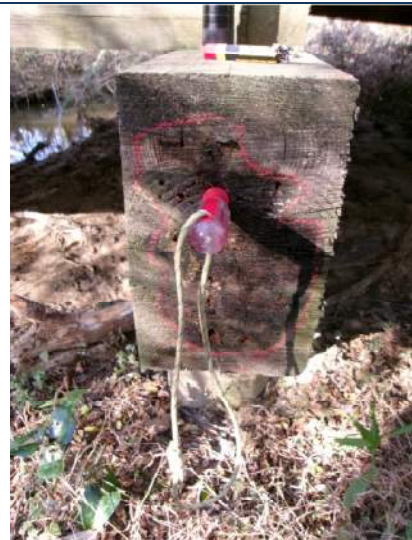
Rot in end of Bent 3 right cap
