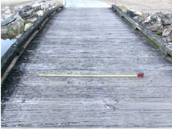
Typical area of deck boards with moderate abrasion
