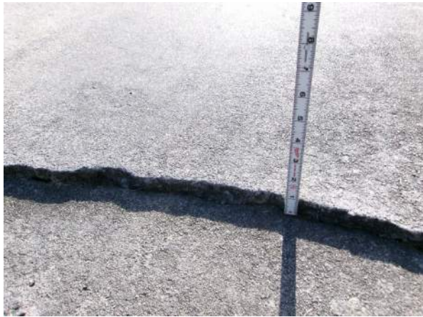
Settlement in approach span at Bent 1
