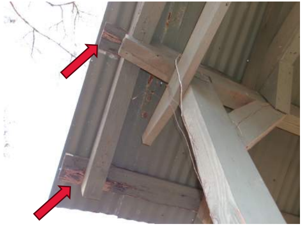
Rot in roof timber members
