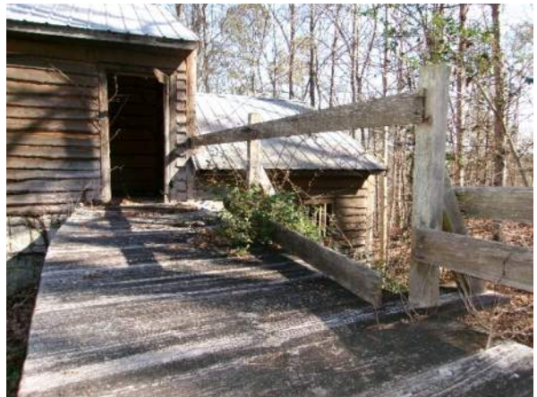
Failing handrail elements
