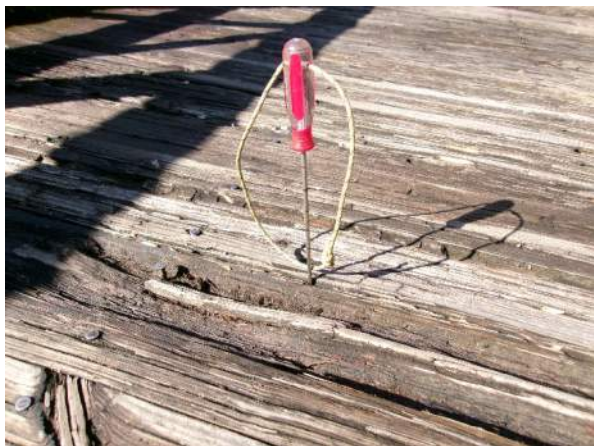
Section loss and rot of deck boards
