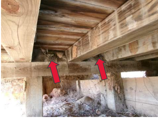
Dirt building up on top of intermediate bent caps along bridge centerline
