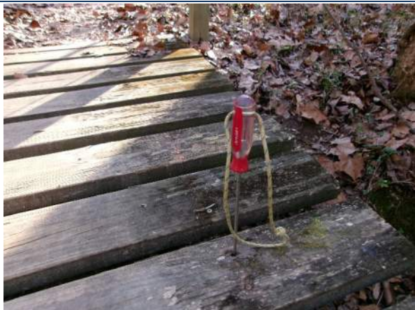
Soft areas in top of deck boards along the edges of the deck, up to 1" awl penetration
