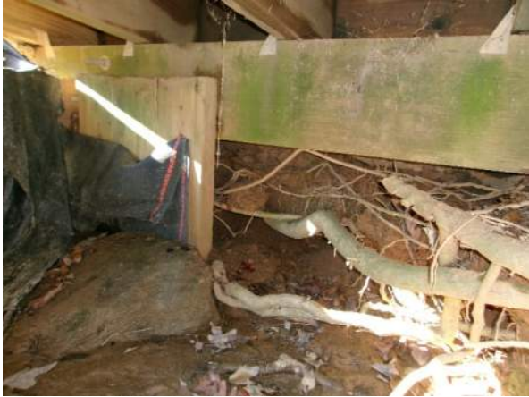
Void behind back wall at Bent 6 with roots extending out from void
