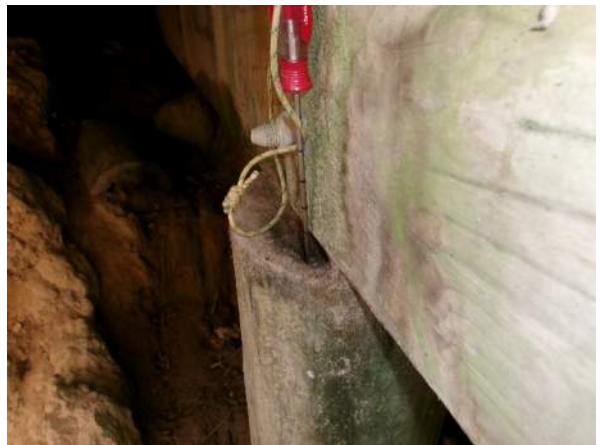
Soft area in top of piles with up to 1" of awl penetration (Bent 8 Pile 2 shown)
