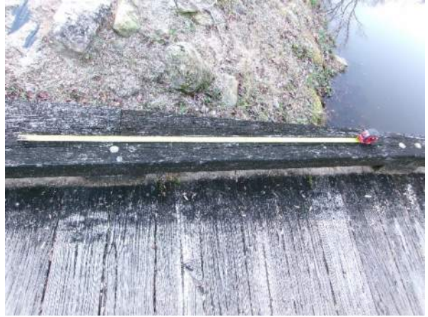
Typical splits and mold along top of brush curbs
