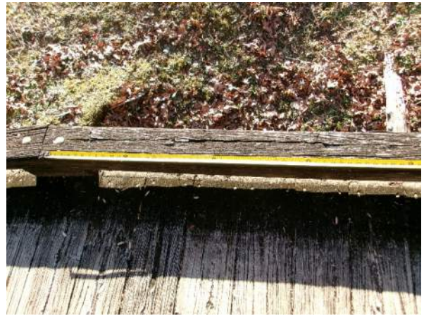
Typical splits and rot along top of brush curbs
