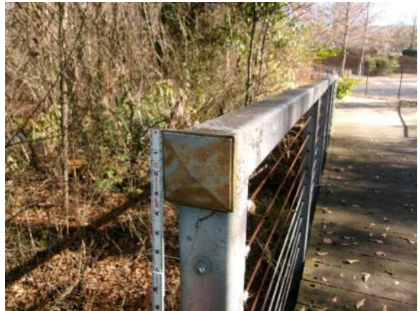
Surface corrosion forming on end caps of handrail
