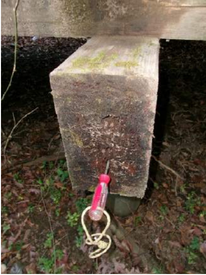
Rot in end of Bent 4 right cap, note the moss growth
