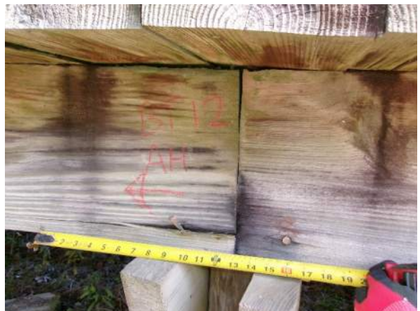
Typical of toenail in exterior beams at bent caps
