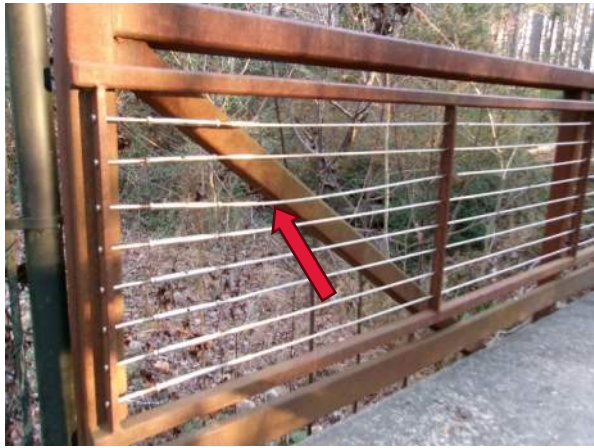
Loose steel cables of railing along left side of bridge
