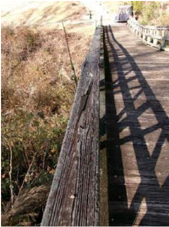
Splitting and rotting of handrail top board
