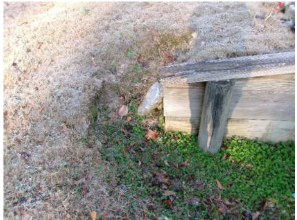
Typical scour hole forming at ends of wing walls at Bent 1
