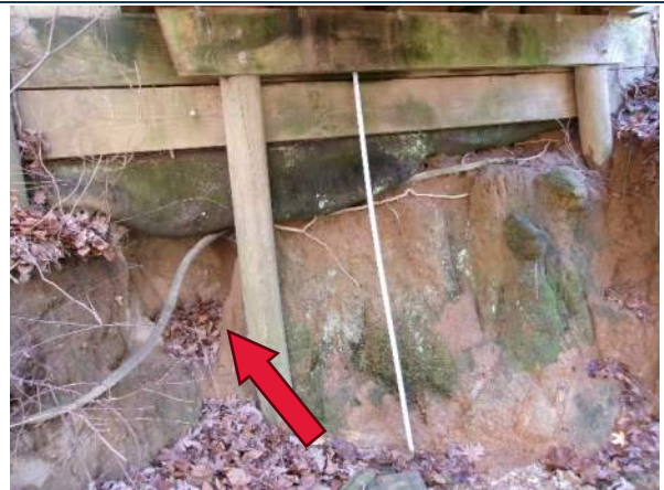
Erosion of endroll at Bent 1 (looking back), red arrow points to 2'-0" diameter hole at Pile 2
