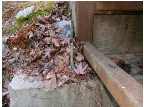
Dirt and debris washing onto the top of the bent caps
