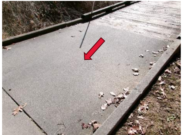
Approach slab at Bent 1 cracking with differential settlement
