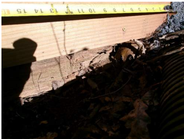
Rot and section loss in left exterior beam at beginning of structure
