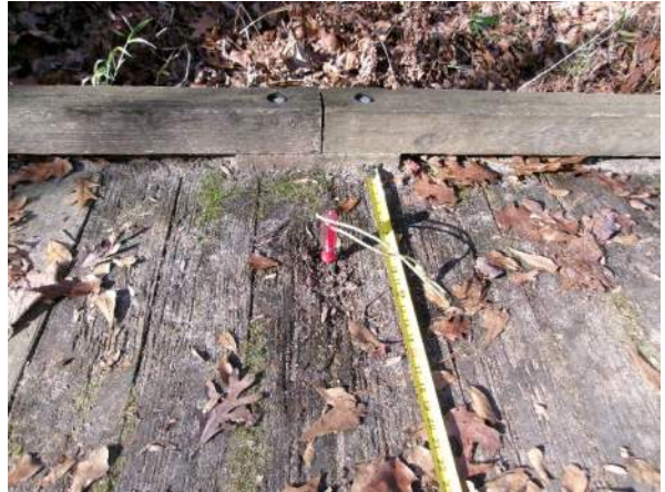
Rot and section loss in deck board along left brush curb at midspan of structure
