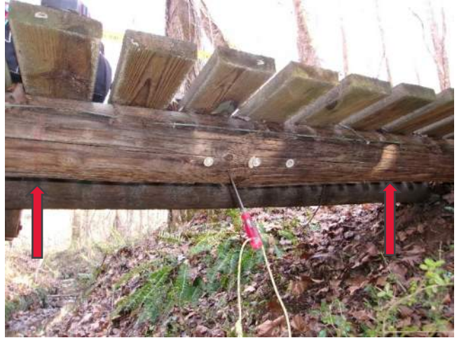
Split in Beam 1 with 1" awl penetration (red arrows mark limit of hollow sounding area in beam)
