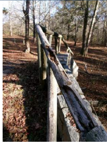
Rot and section loss in top of handrail at right approach
