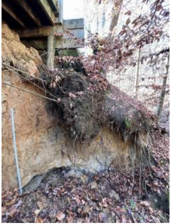
Soil failure at Bent 8
