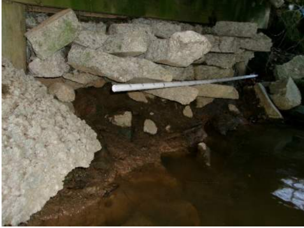
Scour/bank erosion occurring under rip rap/stacked concrete
