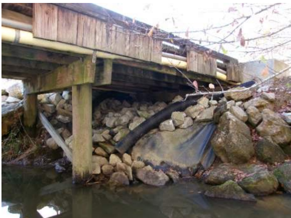
Rip rap missing exposing filter fabric
