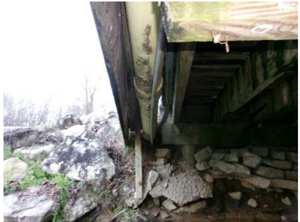
Utilities along left side of bridge deck
