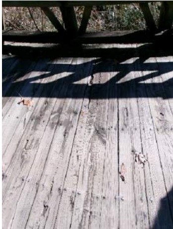
Typical area of deck boards with minor abrasion
