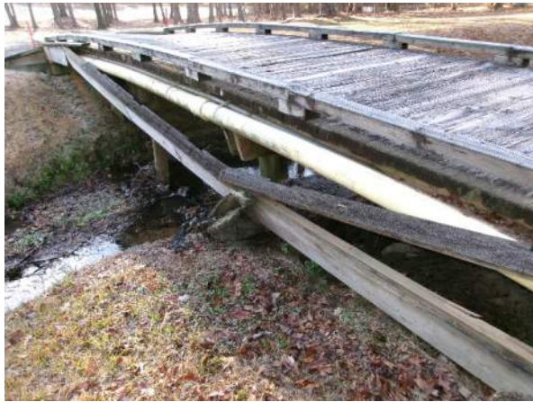
Timber utility façade failing
