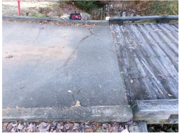
Cracking of approach span at Bent 5
