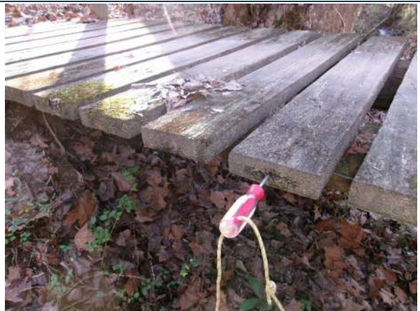
Soft areas in top and edge of deck boards where mold and moss is growing
