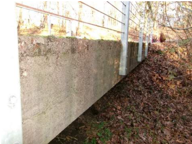
Dirt washing from deck onto Beam 5 in Spans 3 and 4
