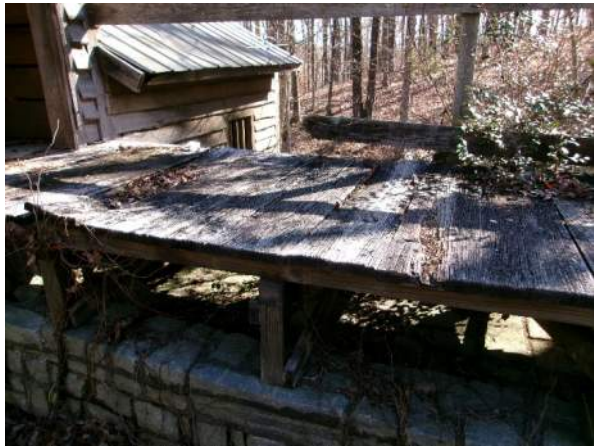
Rotten and failing deck boards in Spans 5-7
