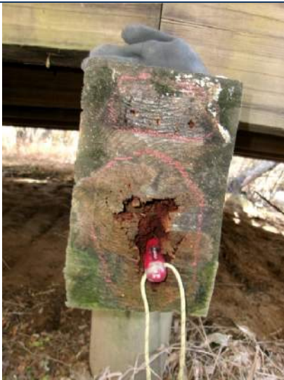
Rot in end of Bent 3 left cap
