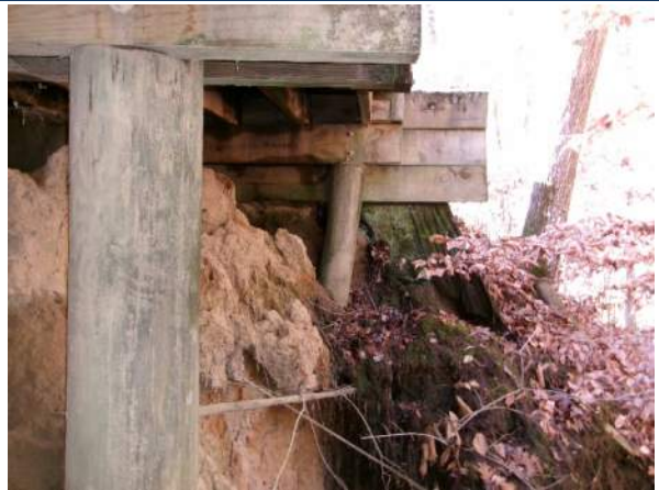
Top of Pile 2 at Bent 8 that is battered outward at the top of pile
