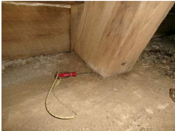
Minor section loss in 6"x6" vertical timbers at the top of the masonry wall
