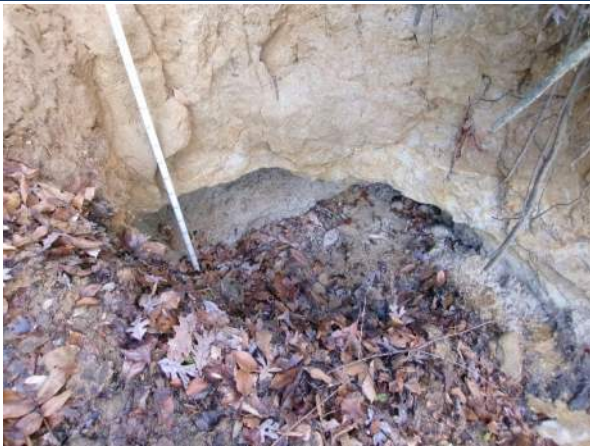
Scour hole forming at the bottom of soil failure between Bents 7 and 8
