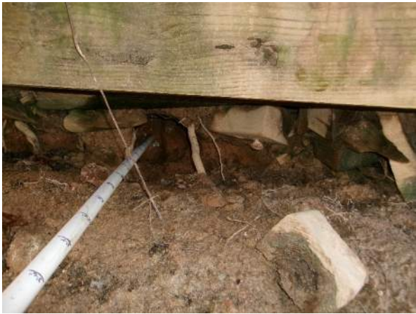
Void under Bent 1
