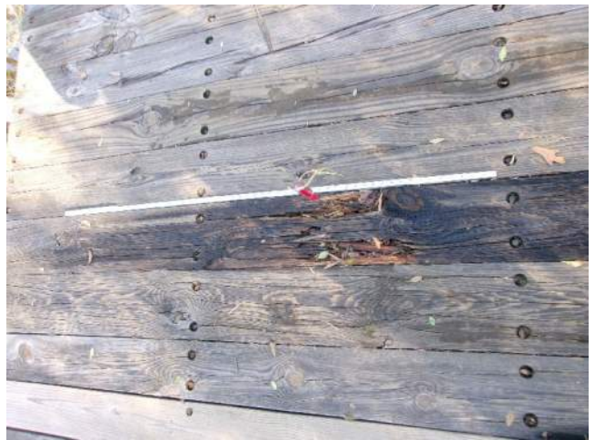
Area of deck board with splits and rot
