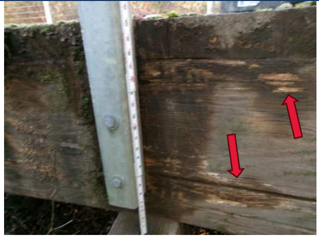
Dirt and moss growth on Beam 5 in Spans 3 and 4 is leading to soft rot
