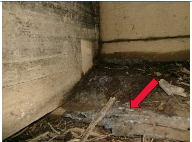
Dirt build up on top of Bent 4 cap, note the white mold
