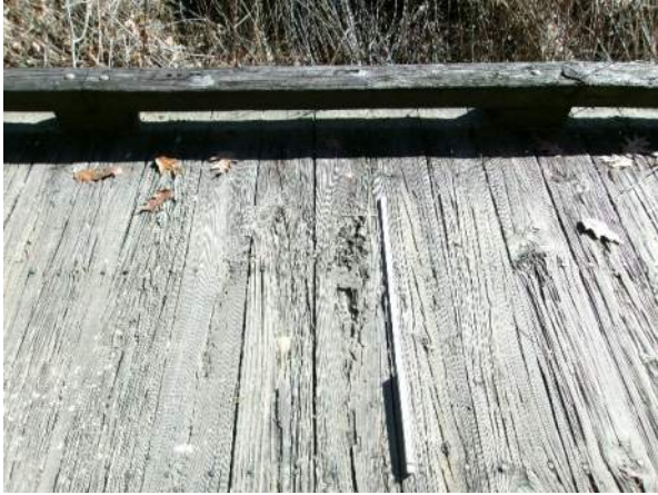
Moderate abrasion on 25% of deck and brush curbs
