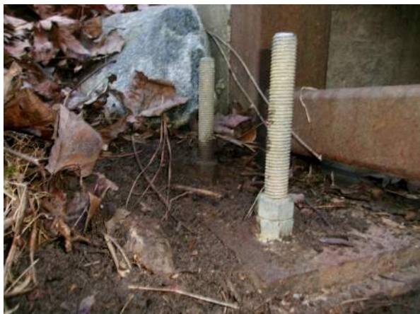
Protective coating of anchor bolts beginning to fail
