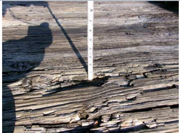
Section loss of deck boards in area with heavy abrasion
