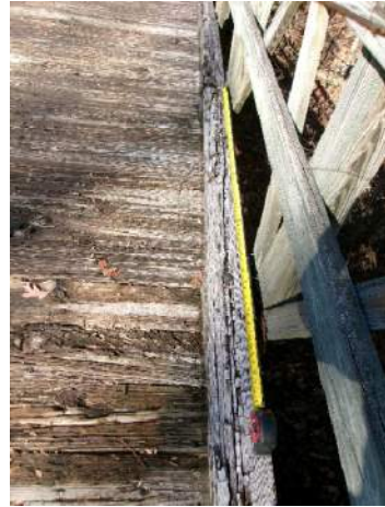
Typical splits and rot along top of brush curbs
