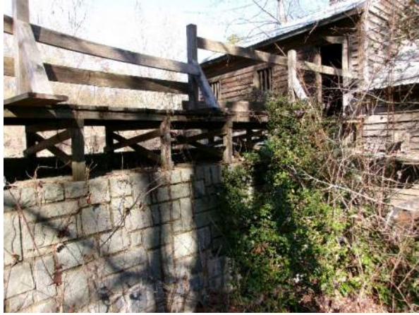
Vegetation growing on right side of masonry wall and substructure elements
