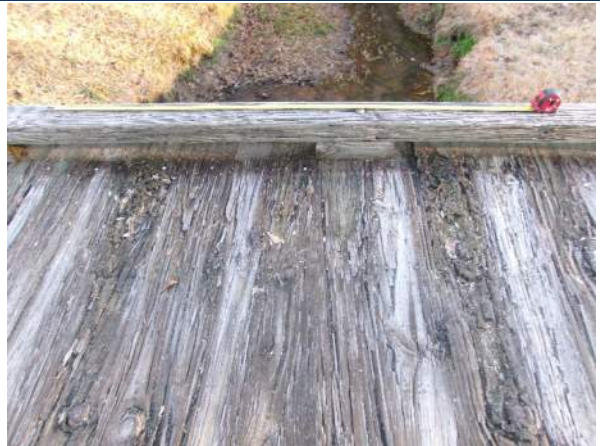
Typical of brush curbs and moderate abrasion of deck boards
