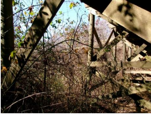
Heavy vegetation along left side of bridge (looking ahead)
