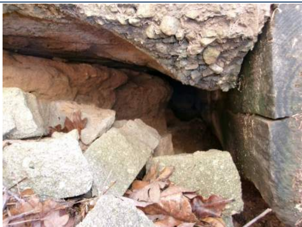
Void behind the back wall at Bent 1 under approach slab
