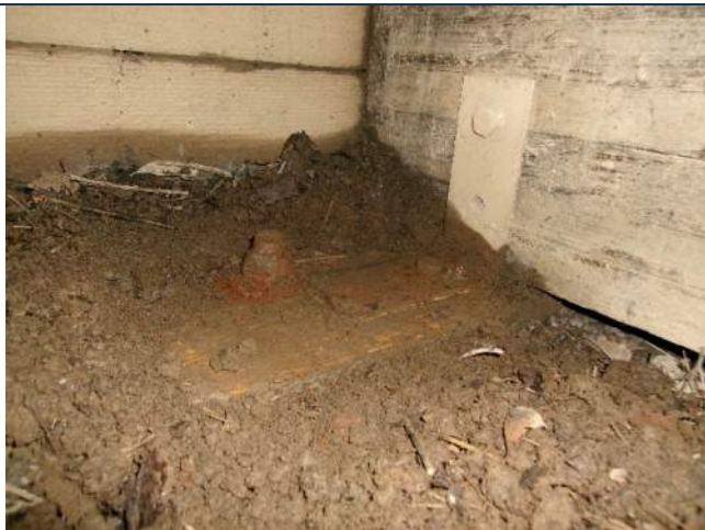
Corrosion of mud sill bolt and angle bolting beam to abutment at Bent 4
