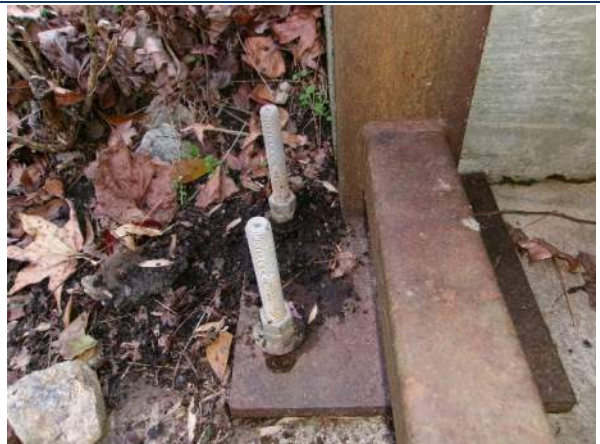
Dirt and debris clogging expansion slots of expansion bearing plates at Bent 2
