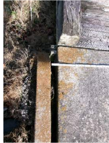
Left curb separating from approach slab at Bent 1
