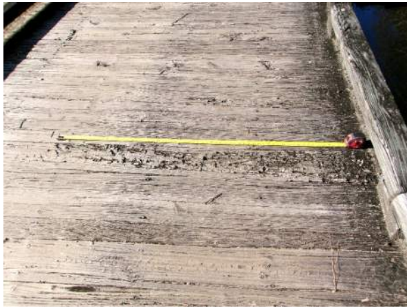
Typical area of deck boards with heavy abrasion
