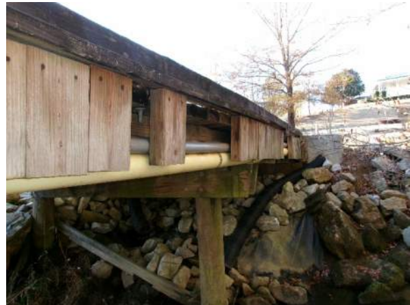
Missing sections of utility façade
