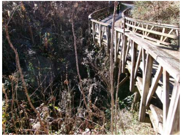
Heavy vegetation growing along both sides of bridge
