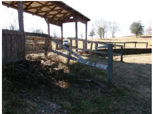
Ramp handrail failing
