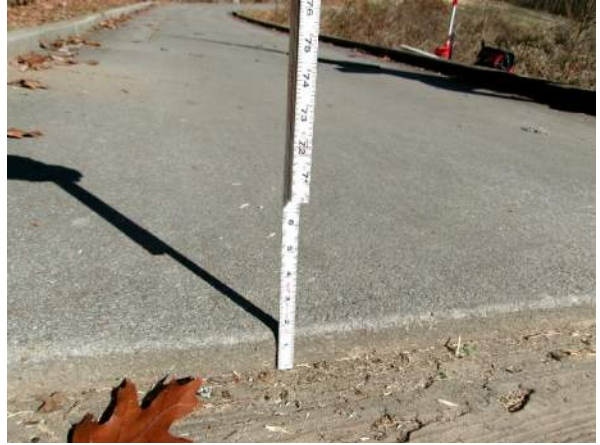
1.5" vertical drop at Bent 1 (looking back)
