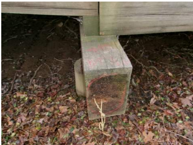
Rot in end of Bent 3 left cap
