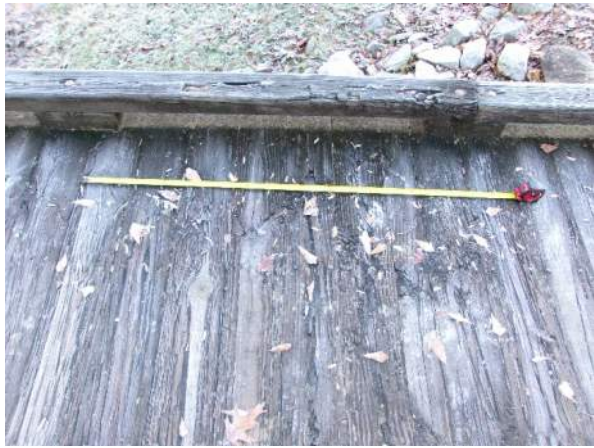
Area of moderate abrasion in Span 4 deck
