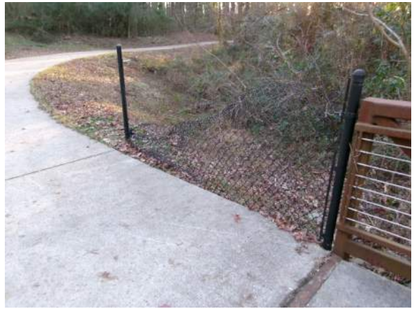
Damaged chain linked fencing at Bent 2 Right
