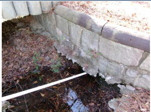
Void and scour hole just down stream from bridge (left masonry wall if looking downstream)
