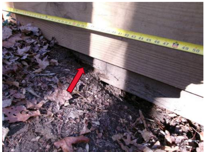
Rot and section loss in left exterior beam at end of structure
