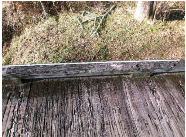
Splitting of brush curbs, this length of curb had a hollow sound when sounded with a hammer
