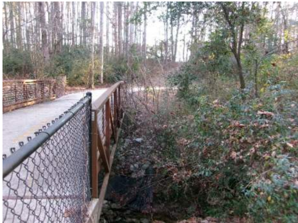
Heavy vegetation growing along both sides of bridge (looking ahead)
