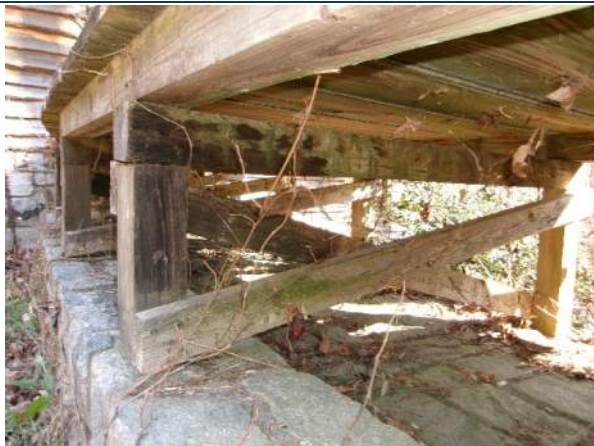
Typical of substructure with mold and mildew on elements
