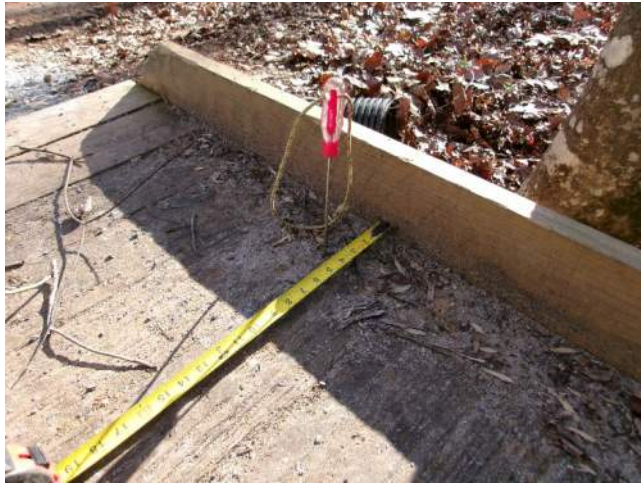
1/2" of awl penetration in areas of soft rot along curb lines
