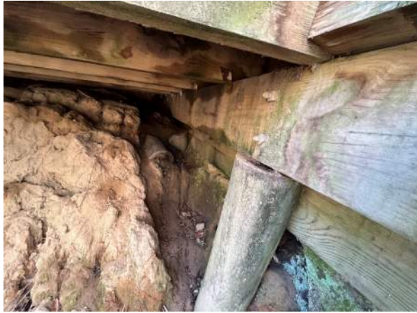
Top of Bent 8, Pile 1 is below grade
