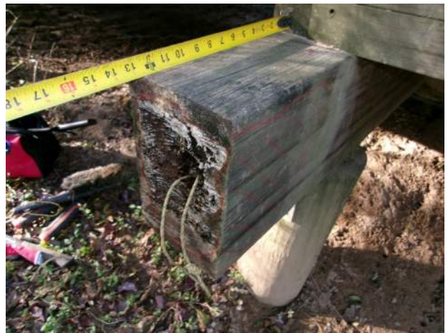
Rot in end of Bent 2 right cap
