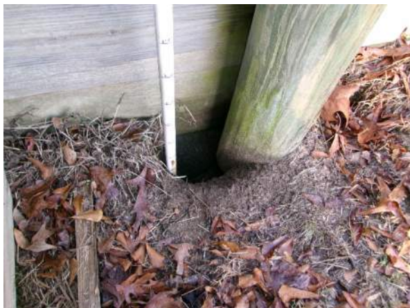
Erosion hole undermining wing wall pile at Bent 1, left
