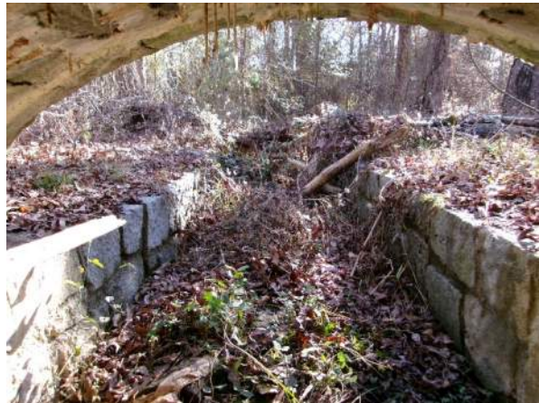
Large debris pile and vegetation downstream of culvert
