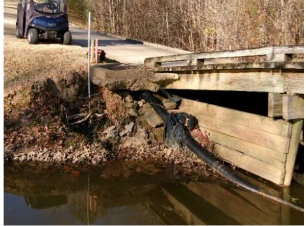
Bank erosion/scour forming below clogged drop inlet at Bent 6
