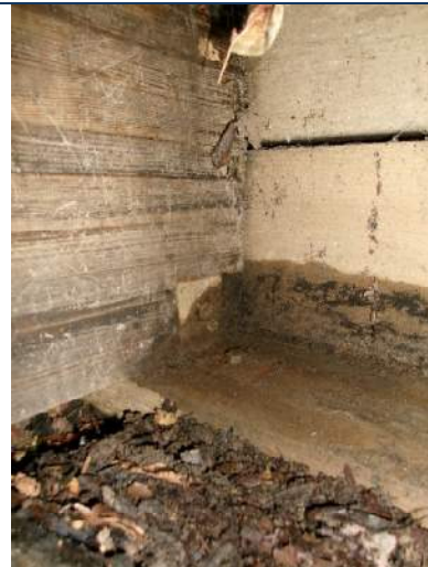
Corrosion forming on steel angle that bolts the beam to the mud sill at Bent 1
