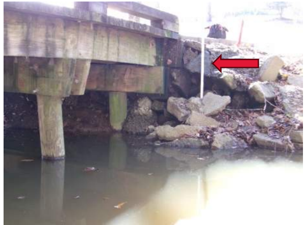
Concrete rip rap added around Bent 4, water is dripping down rip rap from ponding above
