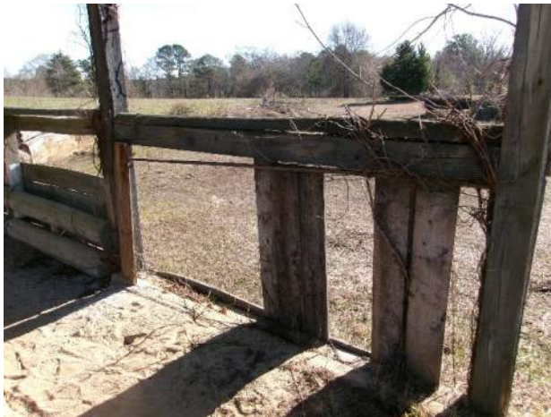
Handrail paneling missing
