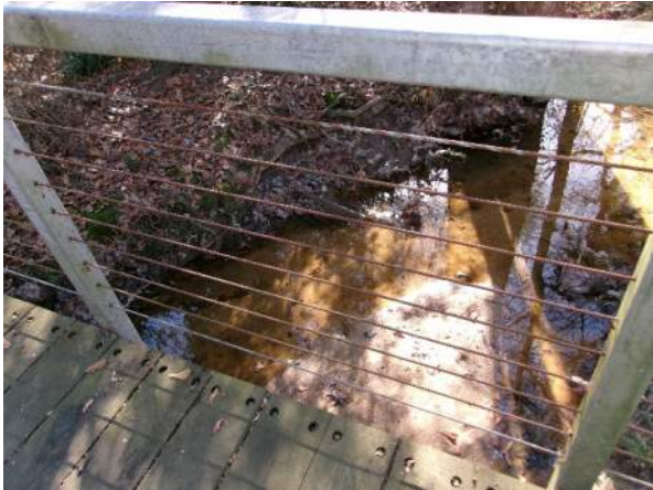
Surface corrosion forming on steel cables of handrail, note the green mildew on vertical posts
