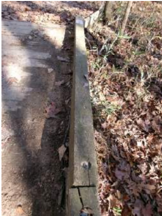
Loose 4"x4" brush curb with missing bolts along right side
