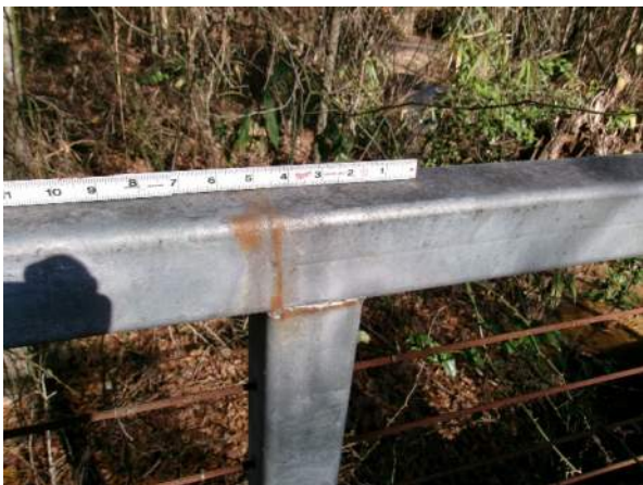
Handrail has localized areas of surface corrosion forming where galvanized coating is beginning to fail
