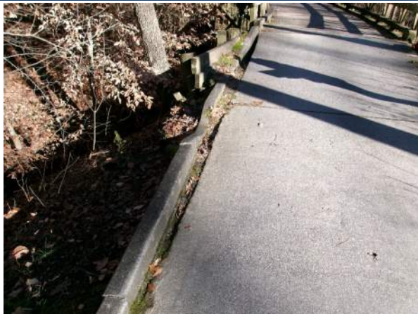
Bent 8 wing wall and curb failing (looking back) Note the oak tree leaning away from bridge
