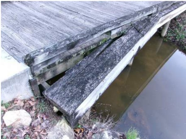
Timber utility façade failing in Span 3
