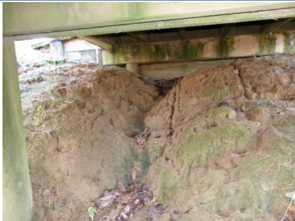
Erosion channel extending from timber backwall at Bent 5 to the stream channel
