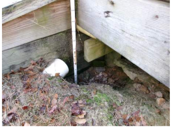
Scour/erosion hole forming below PVC pipe that terminates at the timber backwall of Bent 5
