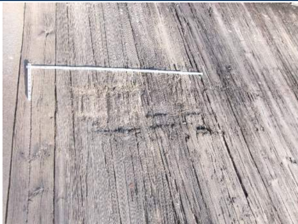
Area of section loss in Span 5 that measures 3'-0" x 2'-0" and up to 1" deep
