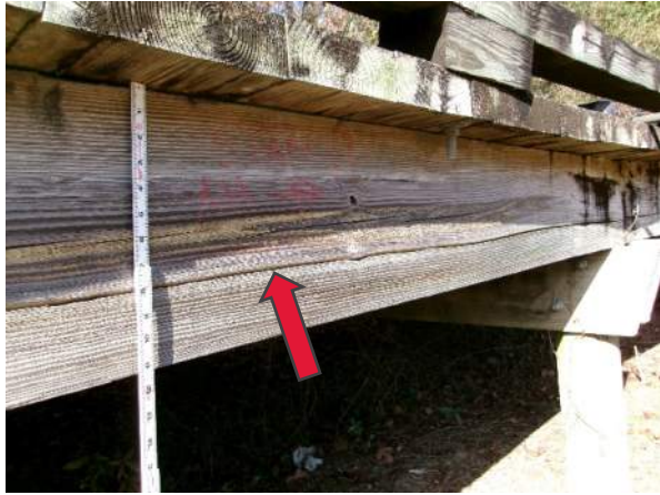
Horizontal split in Beam 6, Span 19
