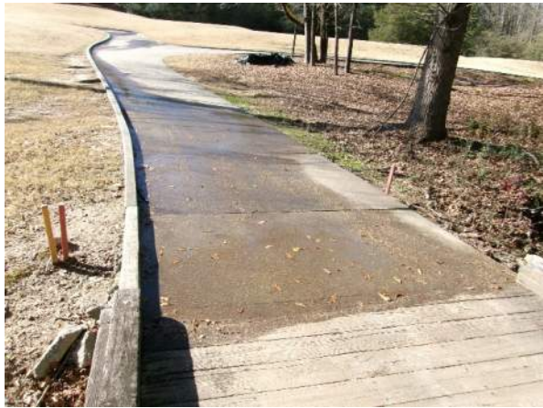
Water ponding at Bent 4
