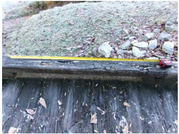
Splitting in top of brush curb in Span 4 left
