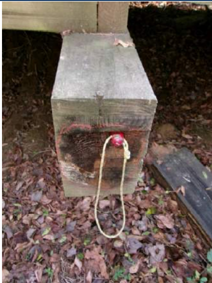
Rot in end of Bent 2 left cap
