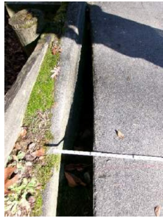
Curb at Bent 8 right failing between concrete pathway
